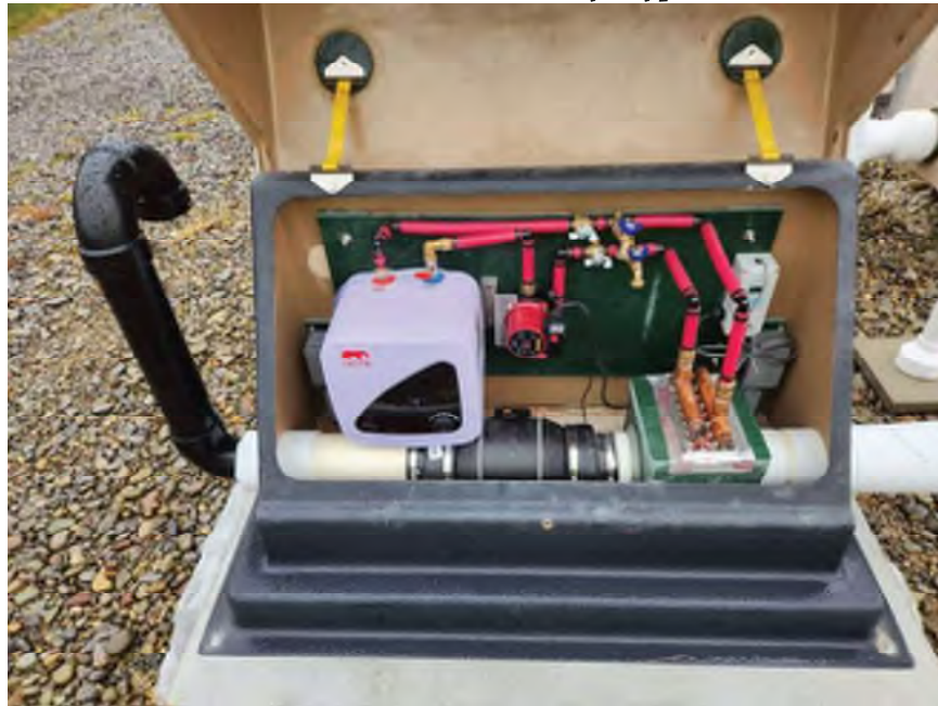
New Blower/Heater Assembly (Typical)
