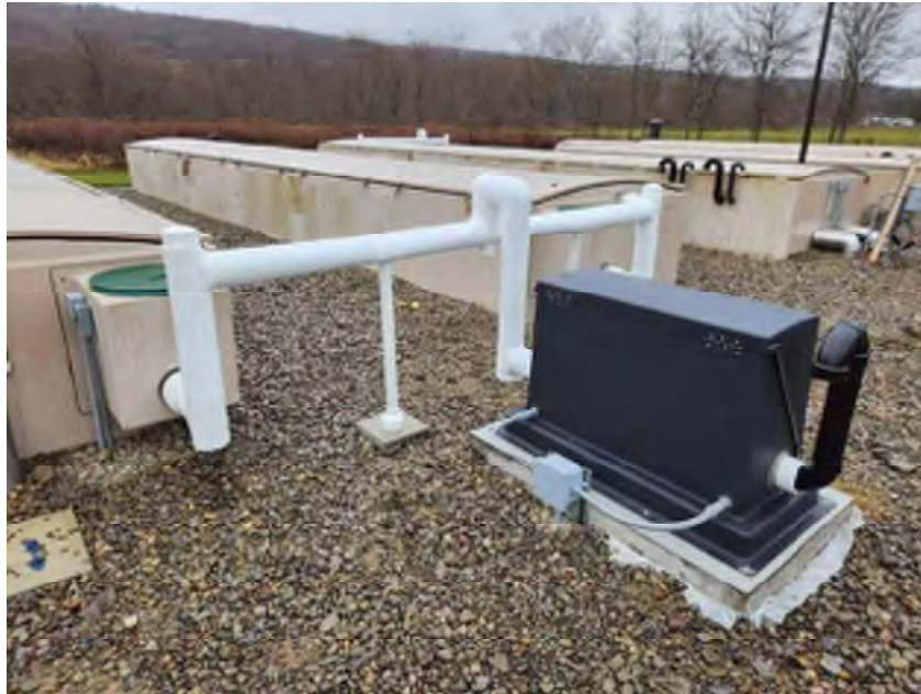
New Blower/Heater Assembly (Typical)
