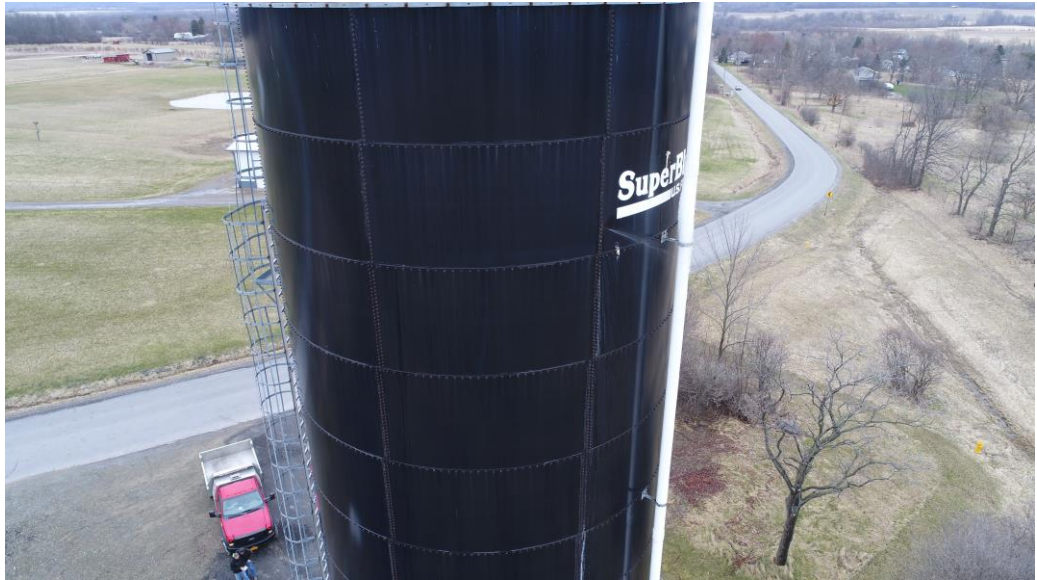
Leak in the tank
