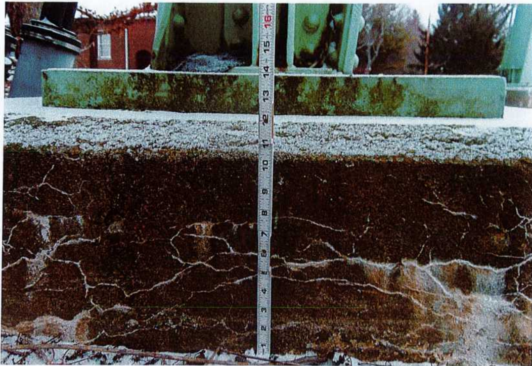
Photo shows the condition of the foundations, which meet the height requirements of AWWA D100-11; 12.7.1: Foundations .
