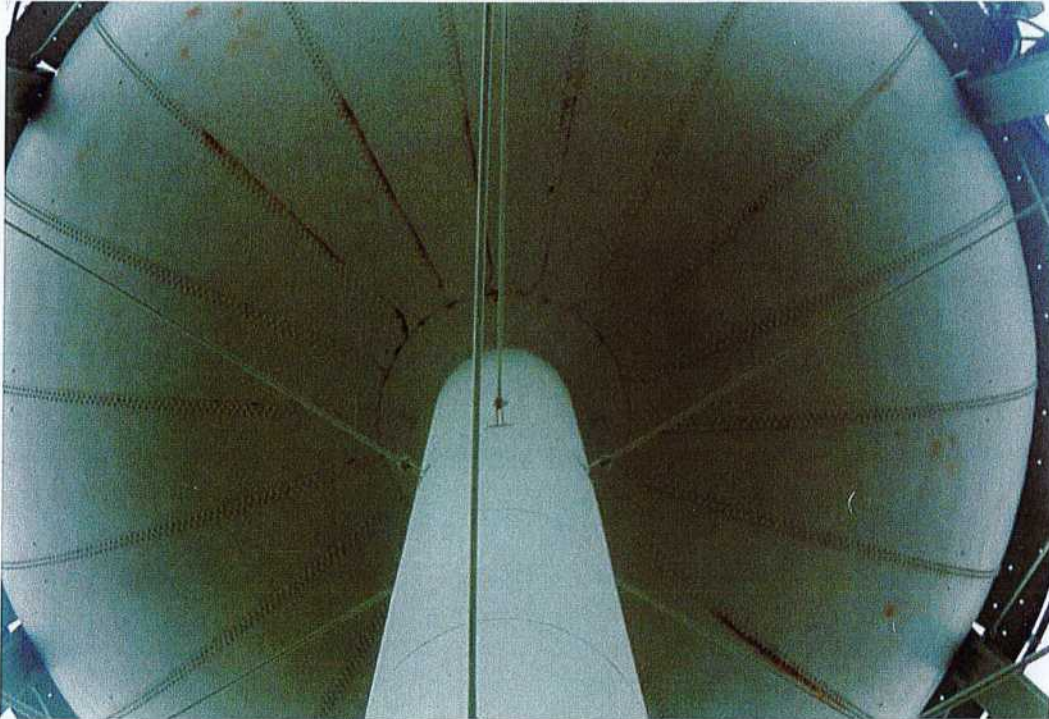
Photo shows the condition of the riser pipe and bowl connection, which appears to be in good condition.
