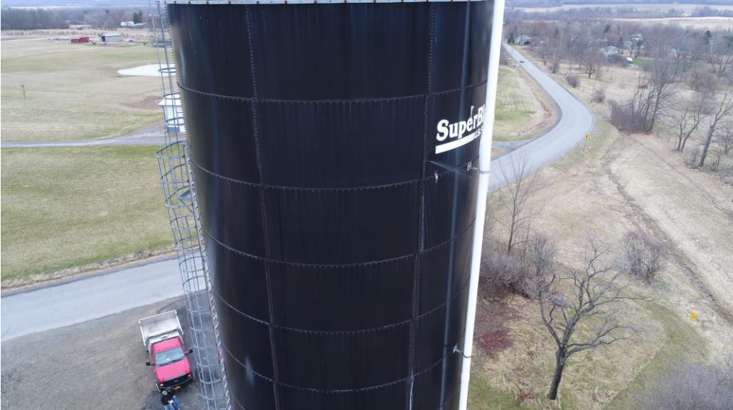
Leak in the tank
