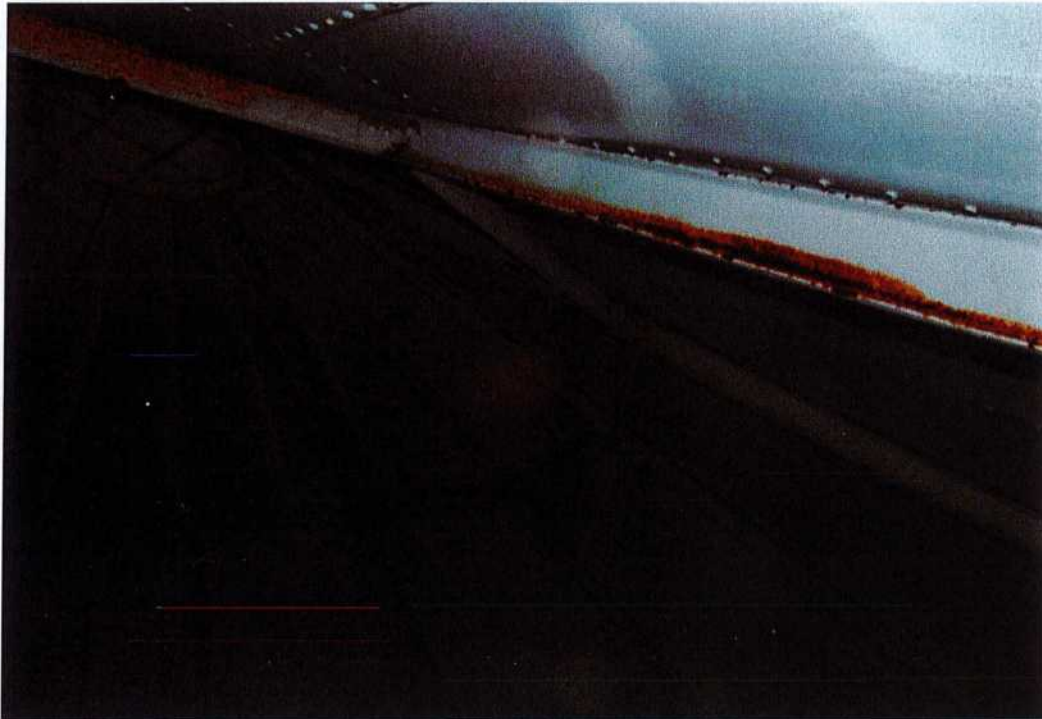
Photo shows the condition of the interior roof. It appears to be in good condition.
