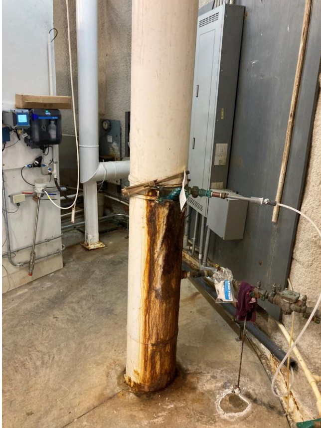
Airport water tank standpipe corrosion at the chlorine injection point.
