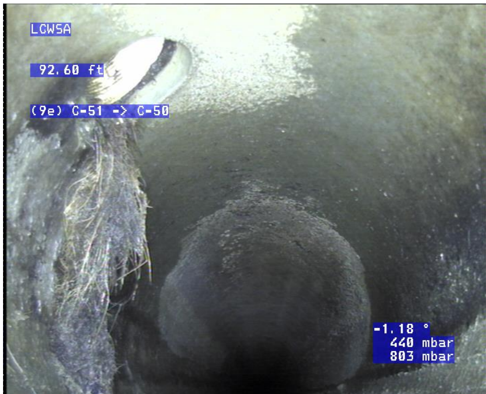
Pictured Below: Roots entering the sewer main at a defective lateral connection to the existing 14" ACP sewer main downstream of PS 9E on East Lake Rd.
